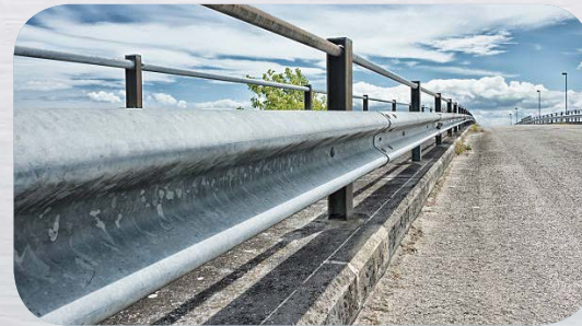
GUARD RAIL BARRIERS
